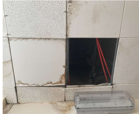
Structural Areas of Concern Photo 3 Water-stained and damaged / missing ceiling finish through water ingress
