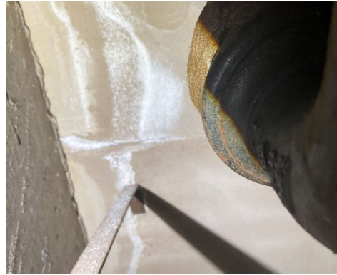
RAAC Observation Photo 3 Penetration through slab, evidence of water ingress at slab edge
