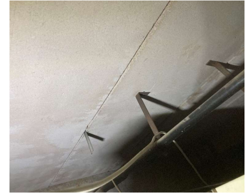
RAAC Observation Photo 7 Suspended grid and services fixed to slab underside
