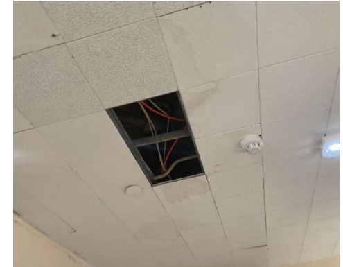
Structural Areas of Concern Photo 7 Water-stained and missing ceiling finish through water ingress
