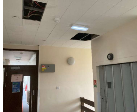
Structural Areas of Concern Photo 5 Water-stained and missing ceiling tiles from excess water ingress
