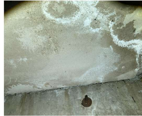
RAAC Observation Photo 5 Extensive water-stained noted throughout
