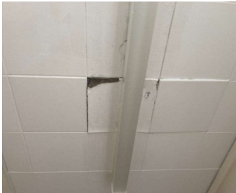
Structural Areas of Concern Photo 4 Water damaged ceiling finish through water ingress
