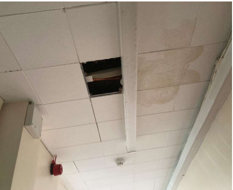
Structural Areas of Concern Photo 2 Water-stained and damaged ceiling finish through water ingress
