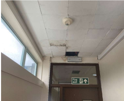
Structural Areas of Concern Photo 1 Water-stained and damaged / missing ceiling tiles resulting from water ingress
