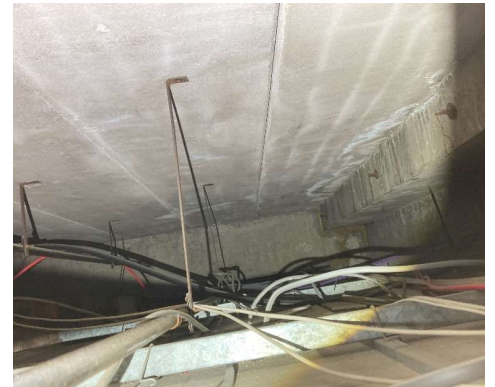
RAAC Observation Photo 8 Minimal coverage of reinforcement with evidence of its location on the surface
