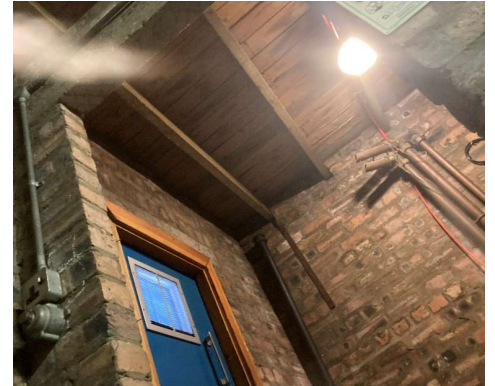
Form of Construction Photo 8 Lift motor room, Timber structure and timber roof deck
