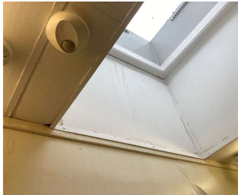
Structural Areas of Concern Photo 6 Water stained and damaged ceiling and wall finish at roof lights
