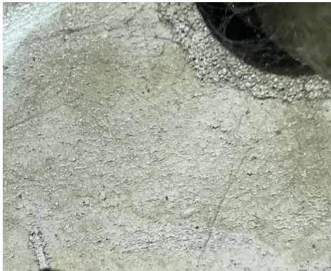
RAAC Observation Photo 4 Penetration through slab
