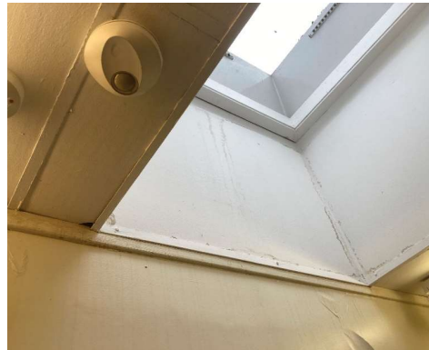
Structural Areas of Concern Photo 6
