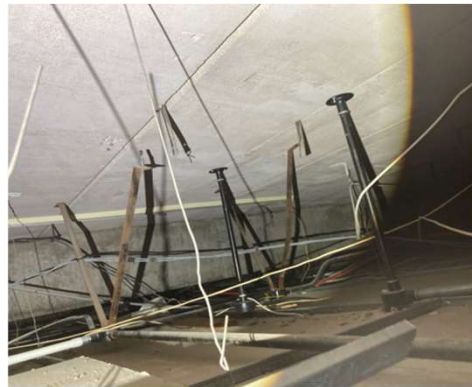
RAAC Observation Photo 6 Failed fixings noted to the slab
