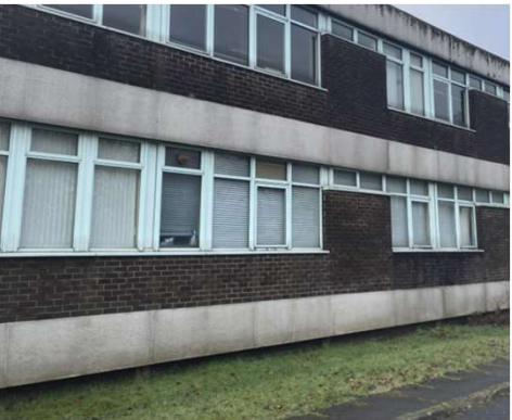
Form of Construction Photo 2 Concrete frame with brick infill, uPVC double glaze windows to the building's front elevation
