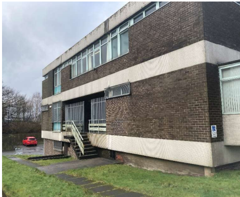
Form of Construction Photo 1 Concrete frame with brick infill, aluminium single glaze windows to the buildings side and rear
