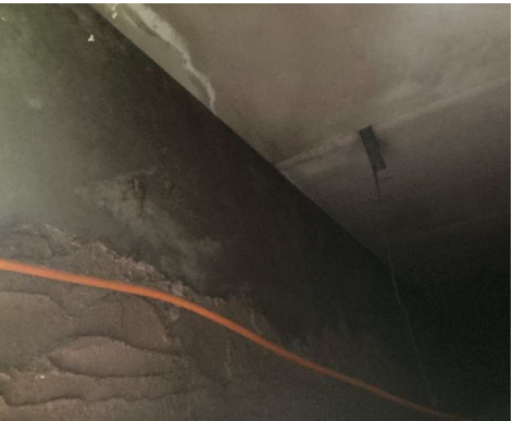
RAAC Observation Photo 2 Water-stained noted at slab edge
