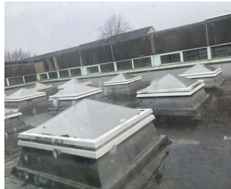
Form of Construction Photo 3 Polycarbonate roof lights with single-ply membrane roof weather covering
