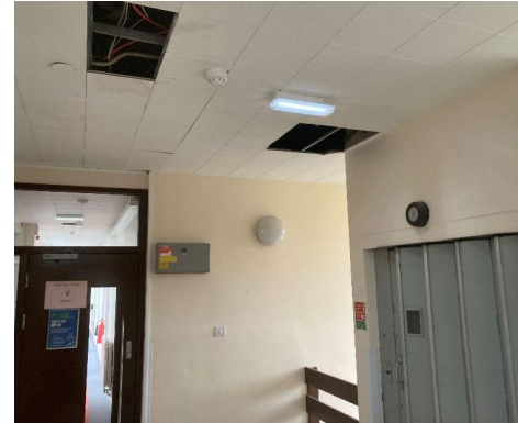
Structural Areas of Concern Photo 5
