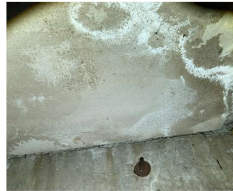
RAAC Observation Photo 5 Extensive water-stained noted throughout
