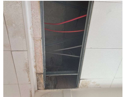
Structural Areas of Concern Photo 8
