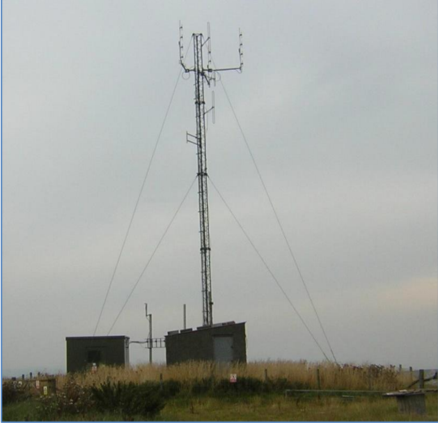
Local Area Broadcast Mast
