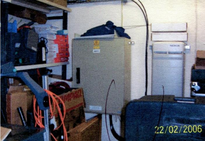
Microcell ancillary equipment within building
