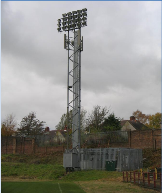
Attached to Floodlight pylon
